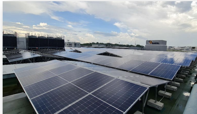
Solar panels at SAESL rooftop
